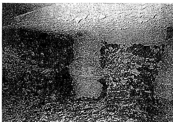
(b) Filled site with clear evidence of ground settlement
