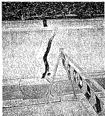
(a) Crack ripping through the concrete
