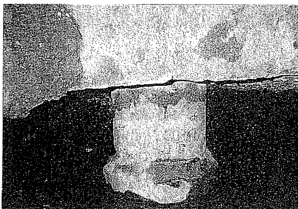
(a) Location where the ground moved laterally by about 150mm
