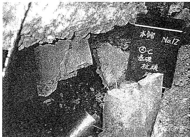
(b) Diameter 350mm PC pile in ordinary ground with liquefaction and lateral spreading.
